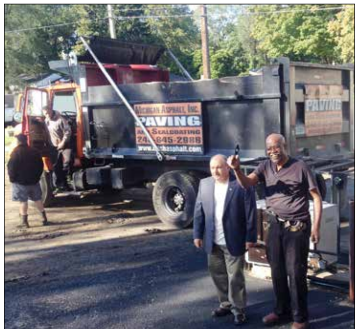
“Happy days are here again.” The Local 5 parking lot is being replaced, with President Troia and Building Superintendent Rev. Willie Anderson delightedly welcoming the paving crew.
